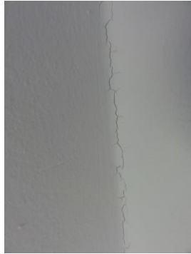
Riss in Badfuge
